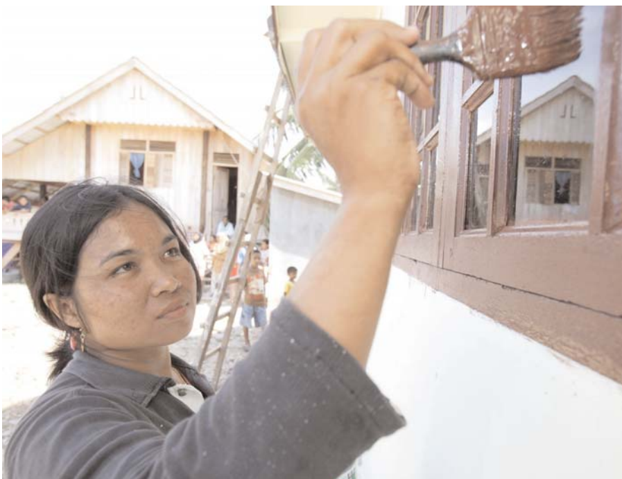
Mahmulia paints a house in the village Beuring In. She was one of 37 women who were trained by Oxfam as house painters in Aceh. This is traditionally a male-dominated area of work, but many of the women found work in the burgeoning construction sector after their training. (Photo: Jim Holmes/Oxfam)
