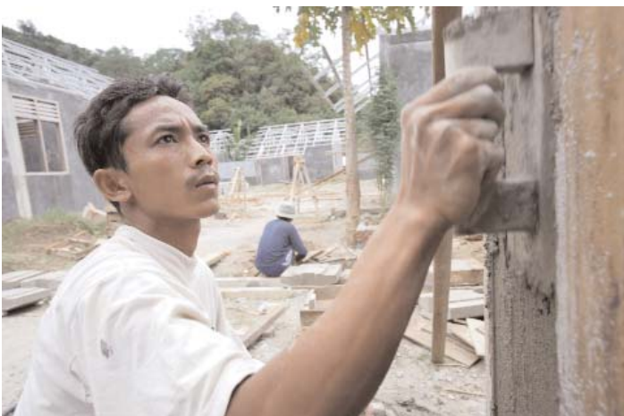
A workman in the process of converting one of the semi-permanent houses constructed by Oxfam in the early phase of the tsunami response to an all-brick structure. We upgraded 549 half-timber houses in this way. (Photo: Jim Holmes/Oxfam)
