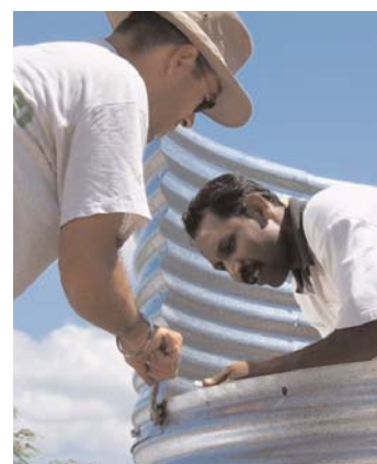
Staff from Oxfam and partner Kinniya Vision construct an 11,000 cubic meter water tank in 'CTB camp', Trincomalee District in the weeks after the tsunami. (Photo: Tori Ray/Oxfam)
